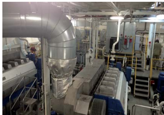
Fig. 13 – Sala macchine. Fig. 13 – Engine room.
