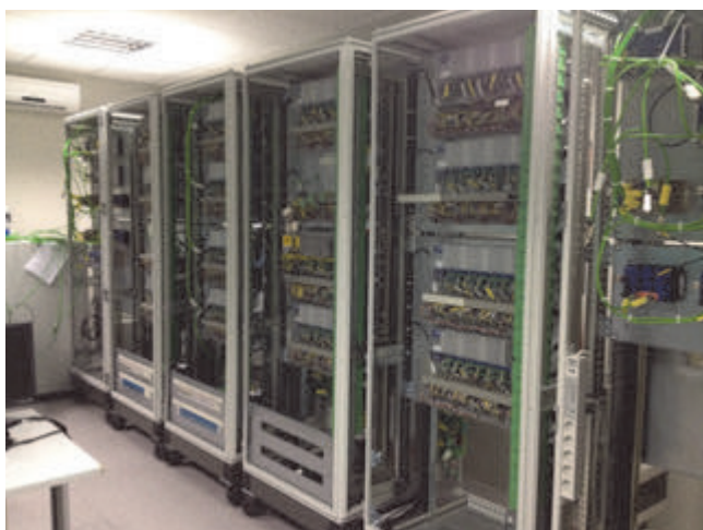
Fig. 5 - Rack con installati i dispositivi del TCMS. Fig. 5 - Rack with the TCMS devices installed.
